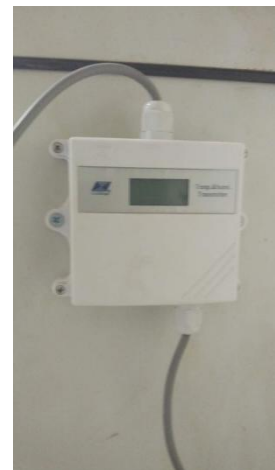
Temp. Humidity Transmitter (in the process supply air)
