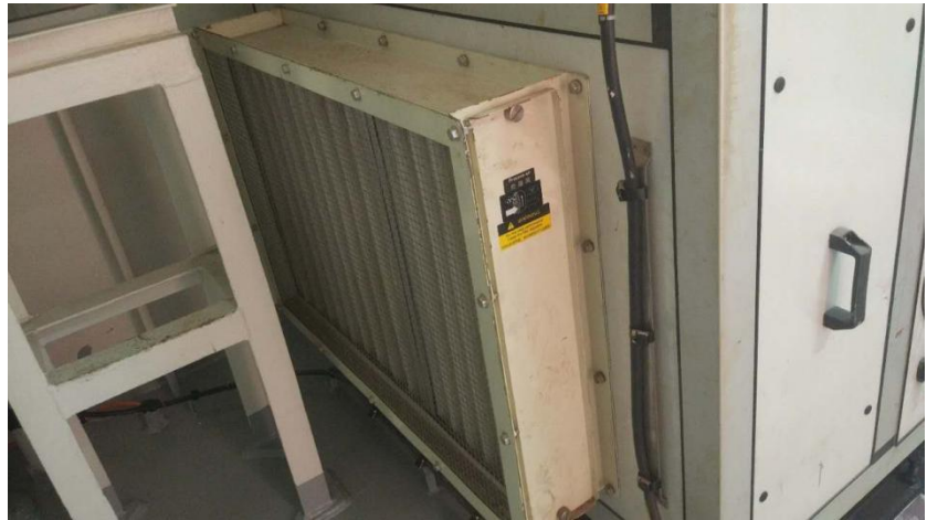
Process air intake
