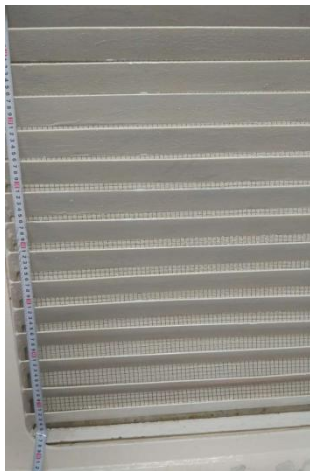
Fresh air intake for the deck house
