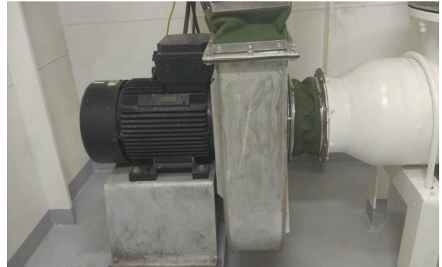
High pressure centrifugal fan(Standby)
