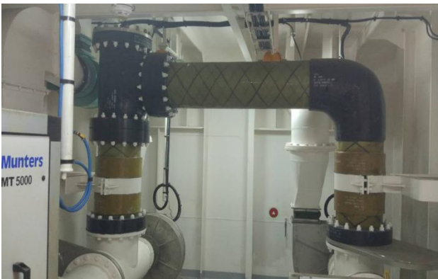
Supply air pipe
